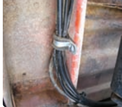
Here are the strobe controllers and harness inside the Bronco, and a typical harness view under the Bronco.
